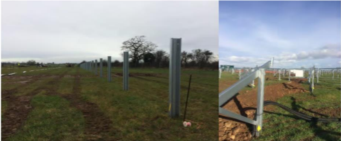
Panel supports (Left), Frames ready for solar panels to be fitted (Right).
