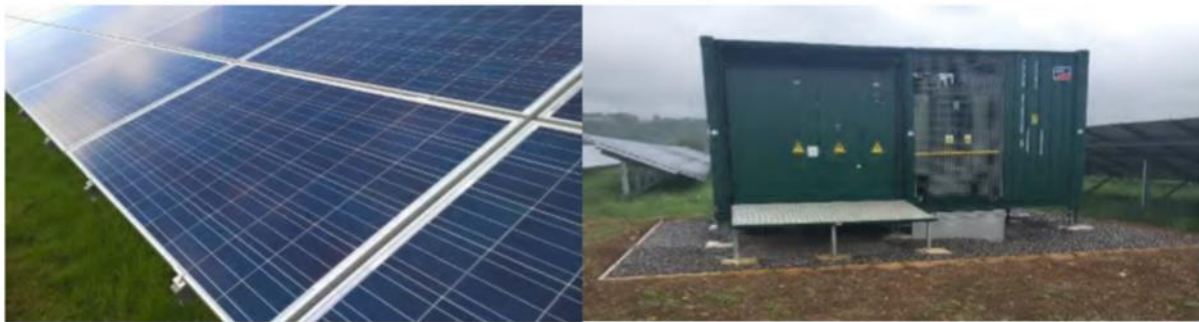
Solar PV Panel (Left), inverter station (Right)
