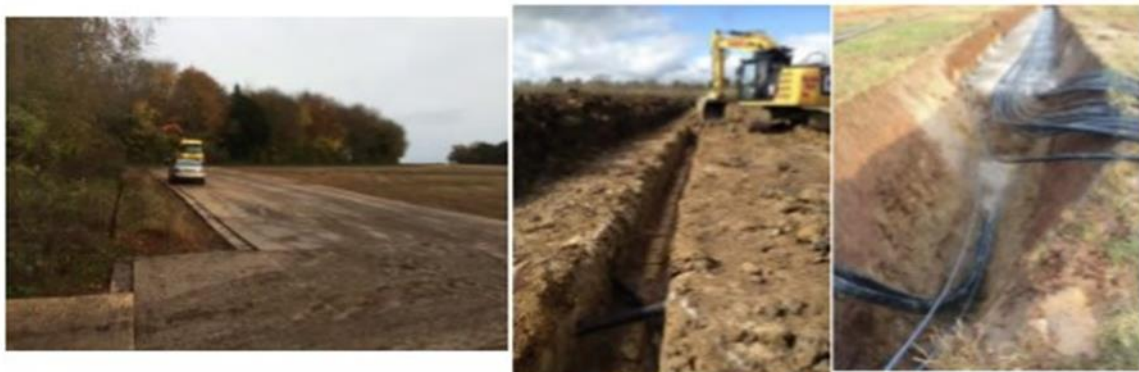
Temporary access tracks similar to those to be used (Left), excavating trenches for cabled (Middle), HV, DC and communications cables in a trench.
