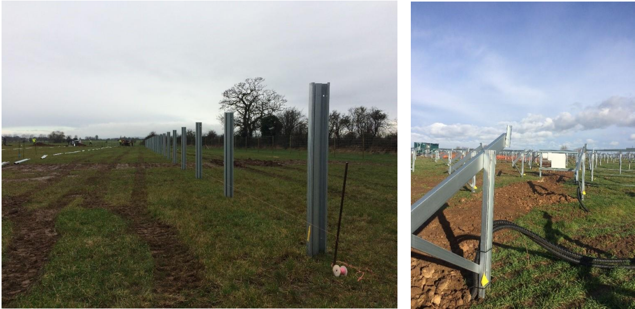
Figure NTS-9: Panel supports (Left) and frames ready for solar panels to be fitted (Right)
