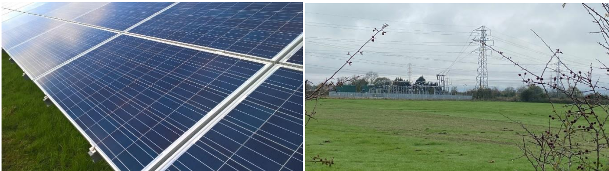
Figure NTS-7: Solar PV Panel (left) and substation with point to connection to 132kV pylon (right)
