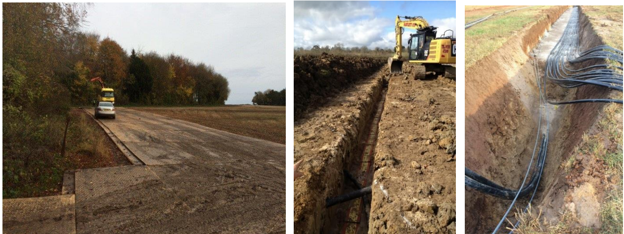
Figure NTS-8: Temporary access tracks, similar to those to be used (left), digging trenches (middle) and HC, DV and communications cables in an excavated trench (right)
