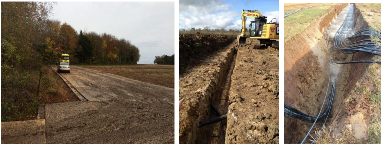
Figure 2-9: Temporary access tracks, similar to those to be used (left), digging trenches (middle) and HC, DV and communications cables in an excavated trench (right)
