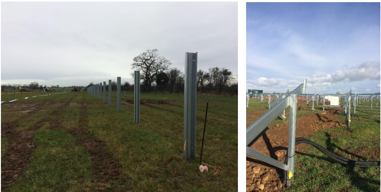
Figure 2-10: Panel supports (Left) and frames ready for solar panels to be fitted (Right)
