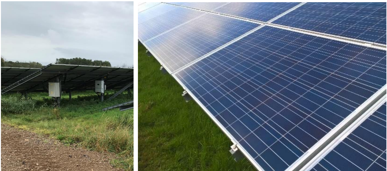
Figure 2-8: String inverters on reverse of PV panel frame (left) and solar PV panels (right)
